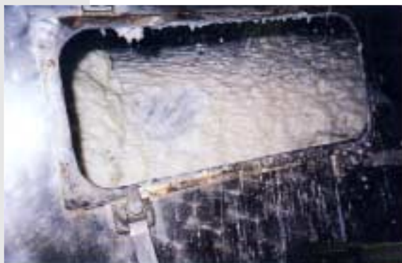
(Before) Build-up of silicate scale on Thune® Dewatering Press.
